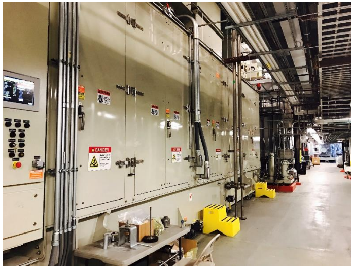
The NYU Langone CHP Gas Turbine Enclosure, courtesy NYU Langone
